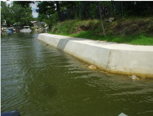
Figure 1. Bulkhead Seawall with no Vegetation
